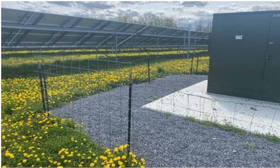
Figure 6. Simple exclusion fence around equipment pad.
