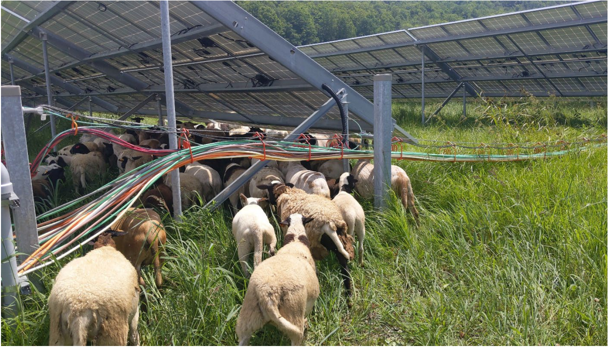
Figure 3. Sheep passing under CAB cabling.
