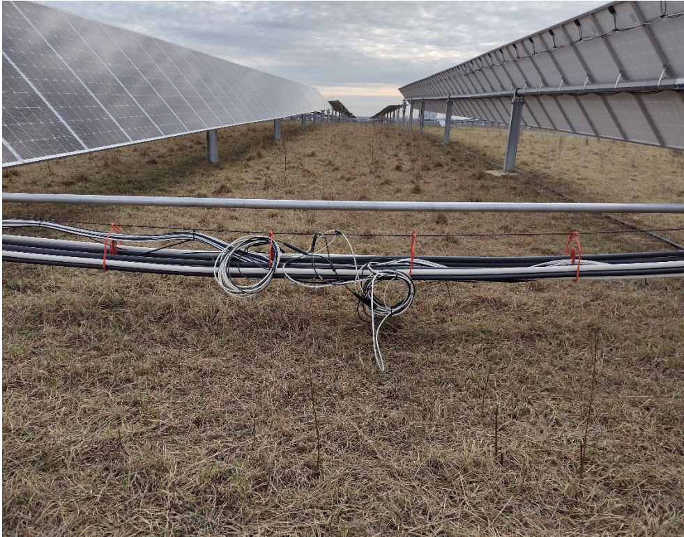
Figure 5. Poor wire management on CAB system, has caused sheep entanglement.
