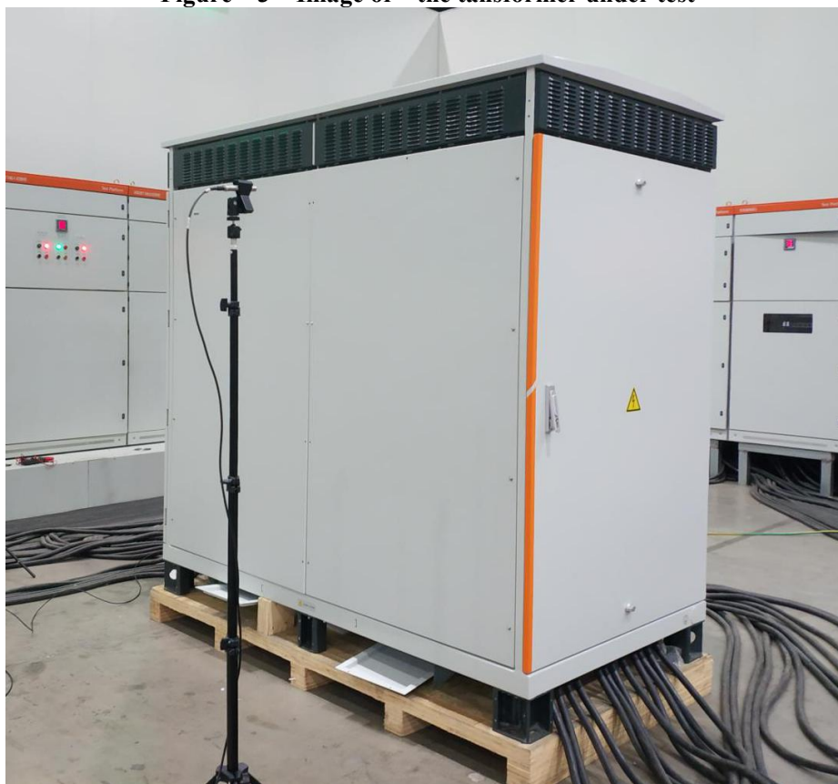
Figure 4 Image of the inverter under test
