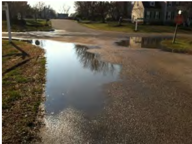
Figure 2.2b. Lack of Gravel Diaphragm
