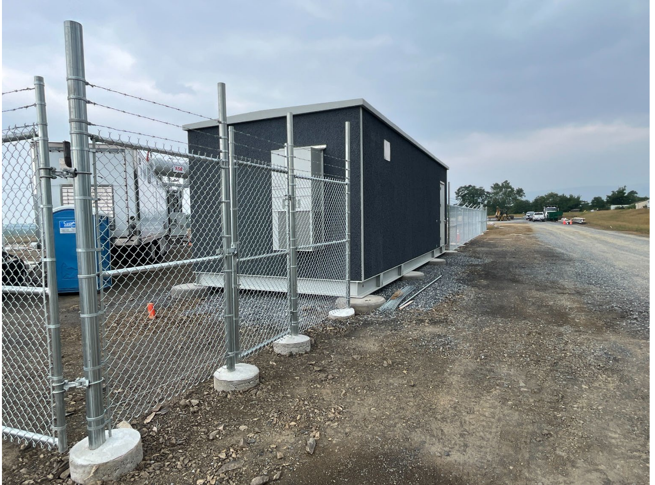
Photo 1. Control Building Example #1
