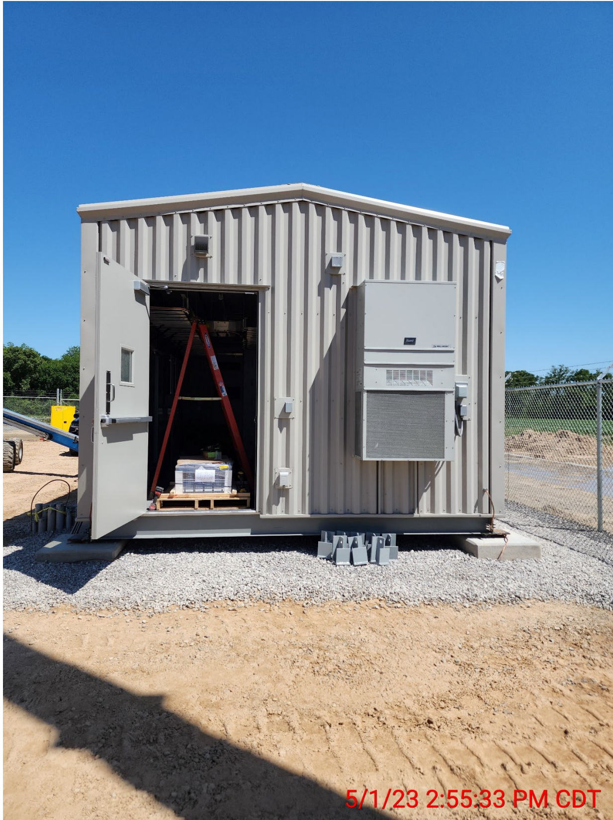
Photo 3. Control Building Example #2
