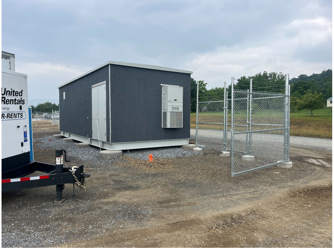
Photo 2. Control Building Example #1
