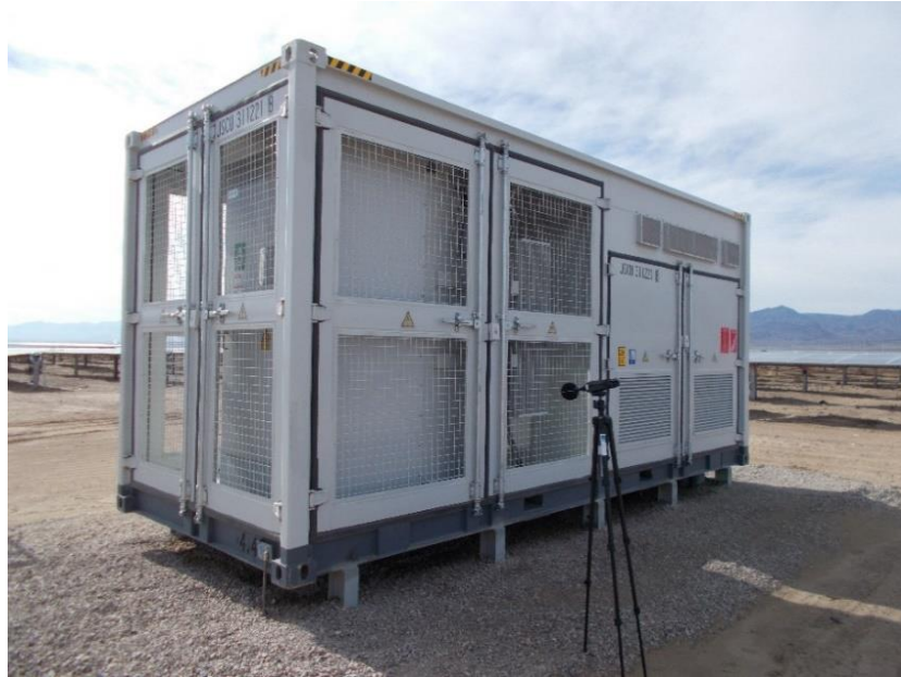
Figure 2: Image of Measurement taken at the Techren Fist Solar Facility of the Sun Grow SG3150U
