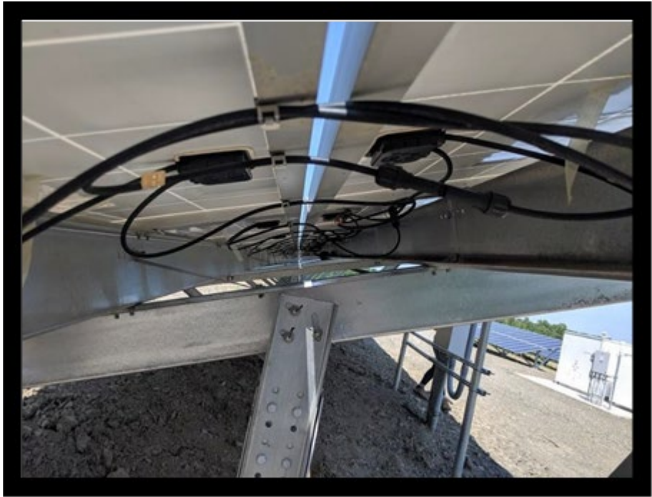
Figure 4. Good wire management on module-module connectors.
